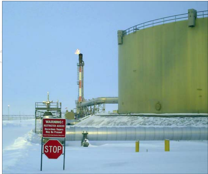
Storage/relief tank at pump station 1—photo courtesy of Ray Elleven
